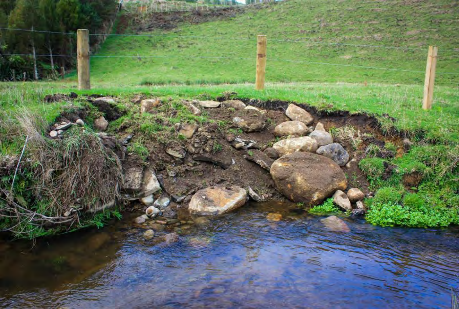
Stream bank erosion
