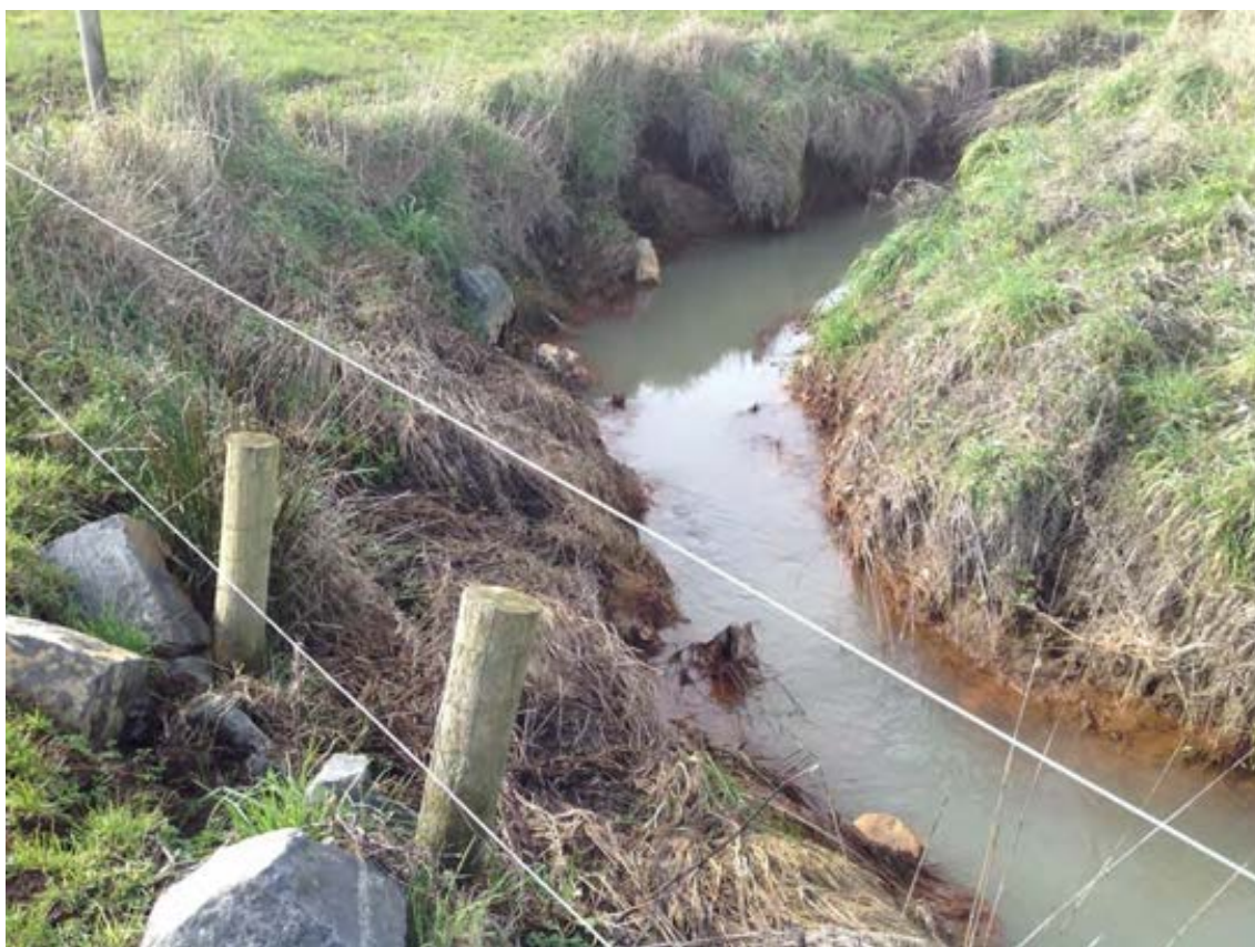
Plate 5: Rock armouring collapsing into the stream
